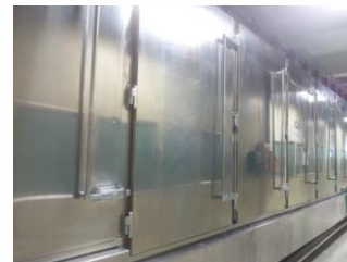
Sterilization cooling / temperature control system
